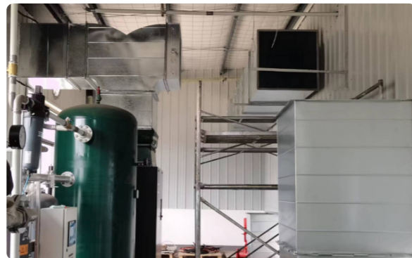
Pipe connecting the heat outlet of the air compressor with the molding room
