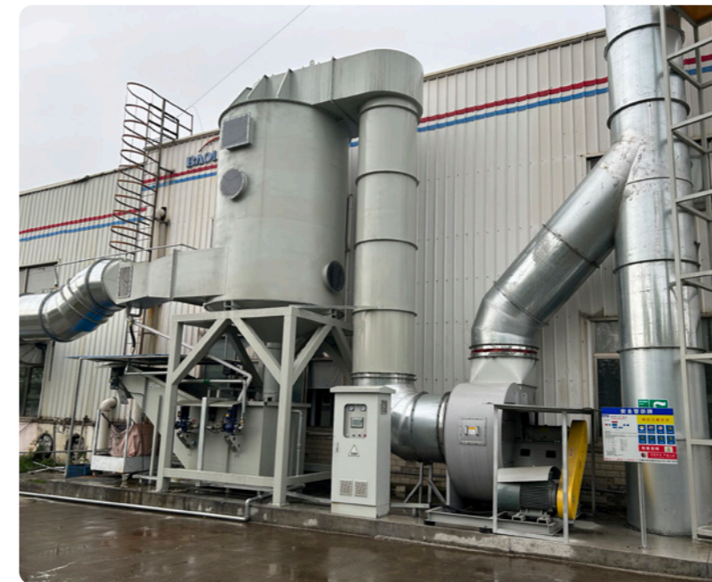
Waste gas control facilities
